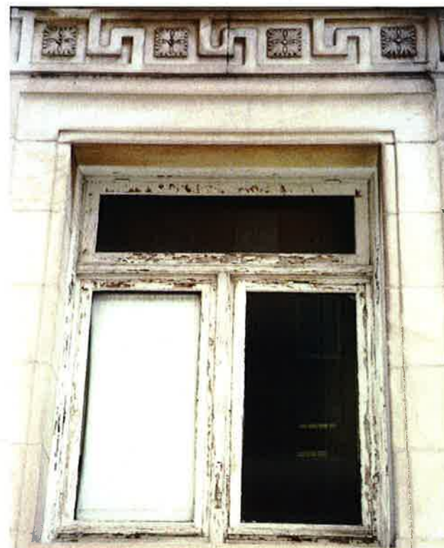
Photograph 15: Paired vertical pivot sash topped by a wide awning transom sash typical for the first floor, 2002.
