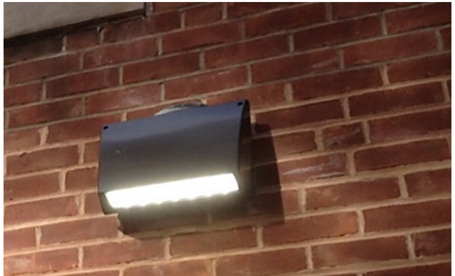
New Wall-Mounted LED Lighting
