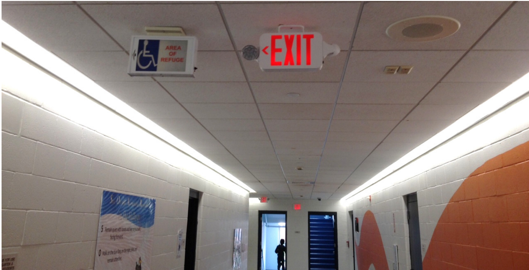
Hallway and EXIT sign LED Lighting
