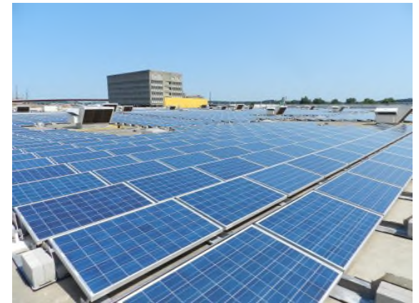
Figure 1. IKEA, which features the largest solar array in the State of Connecticut offers an example of how Long Wharf is already off to a robust start in taking advantage of these opportunities
