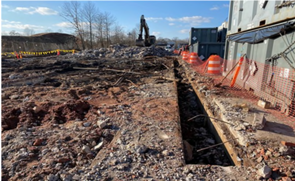
View of pipe removal in the north trench from column 48-40 looking west.
