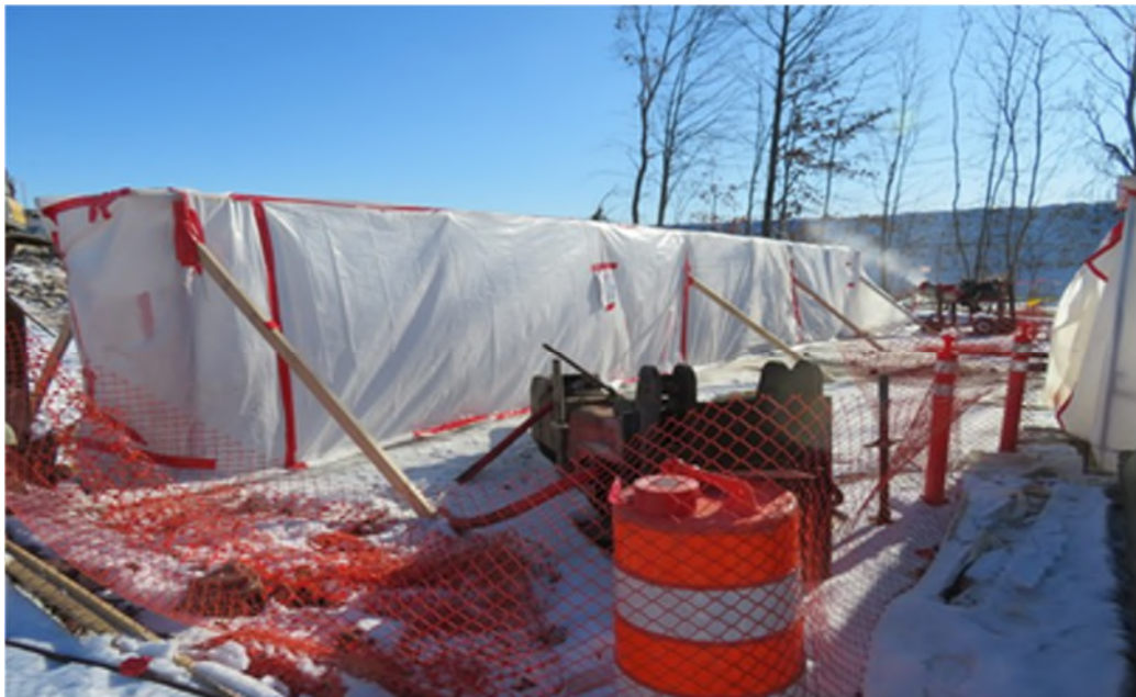
View of scaffolding frame assembled over ACM material in trench at column 33.
