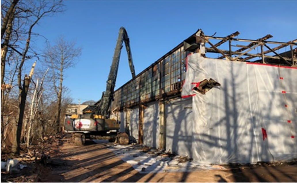
SWC removing roof on southern half of the main building between Columns 14-5.
