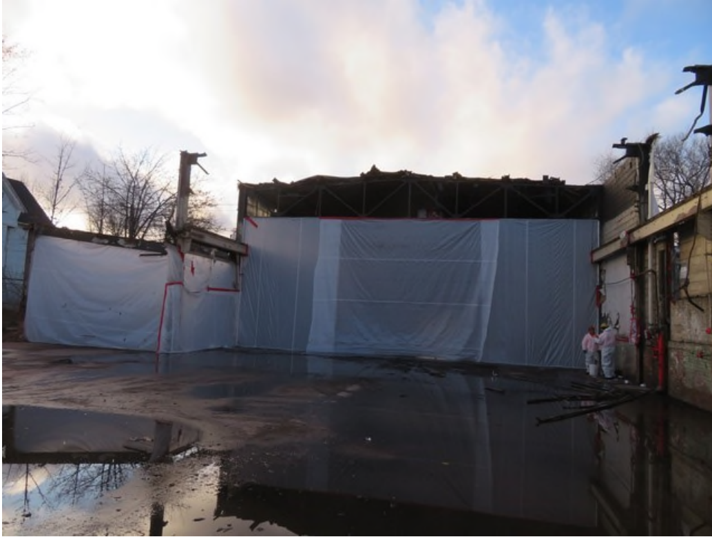
View of critical barrier installed at column #5 for remaining roof debris removal.
